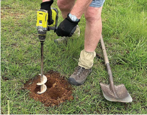
Fig 6.3: Using a drill and 600 mm long auger of 75 mm diameter to drill 3 holes for planting.
