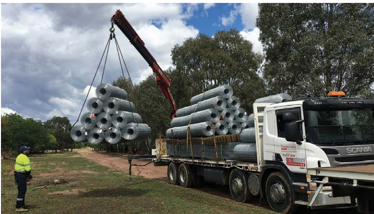
Fig 7.14: Unloading rolls of steel mesh shipped direct from the manufacturer to a central location.
